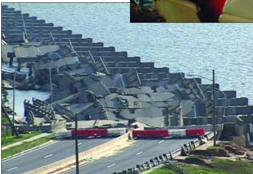
Destruction from Hurricane Katrina.
