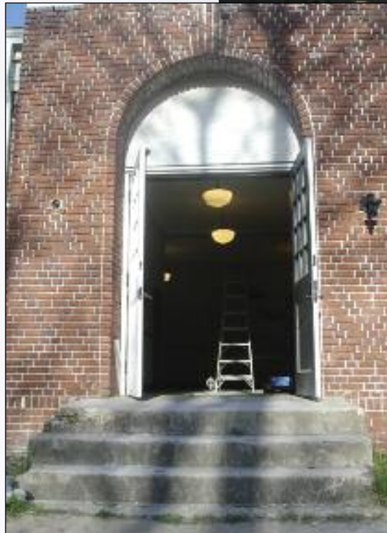
Renovations to the Lil' Red School House in Drew, Miss., are nearing completion. The building, built in 1928, was originally a Rosenwald School, where blacks were educated in the early 1900s.
